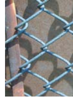
Before: exposed & corroded surface
